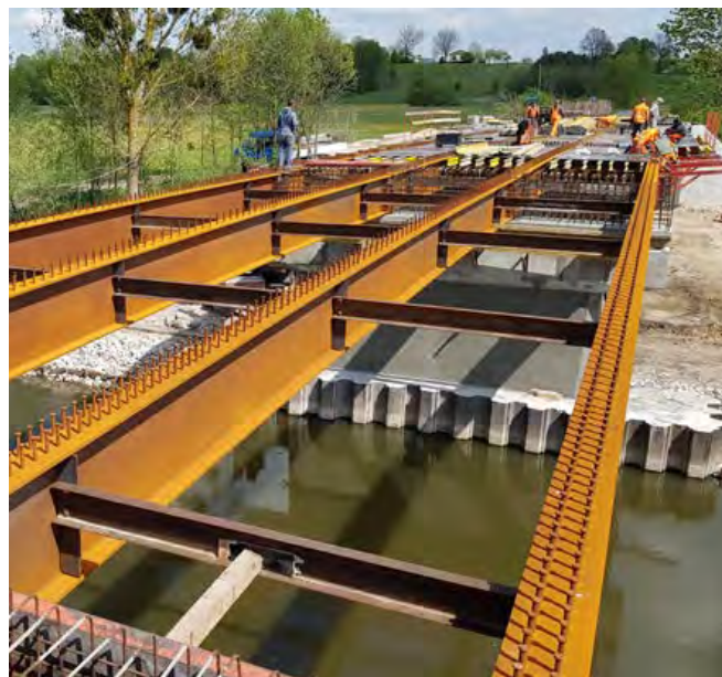
A bridge in Poland built using XCarb™ recycled and renewably produced steel ↑
