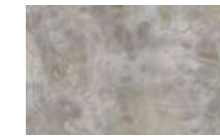
FCC 025 Cracked plaster
