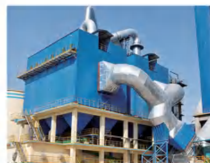
水泥窑头窑尾除尘项目 Dust removal project at the head and tail of cement kiln
