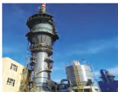
电厂脱硫湿电一体化项目 Power plant desulfurization wet electricity integration project
